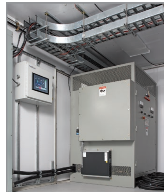
Hydrogen Generator Power Supply
